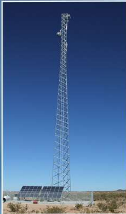
Wireless Telecommunication Towers
