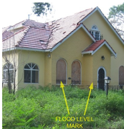
Fig. 10.3 Abandoned home east of 17 th Street Canal, July 2006. Photo courtesy of D. Dickey.
