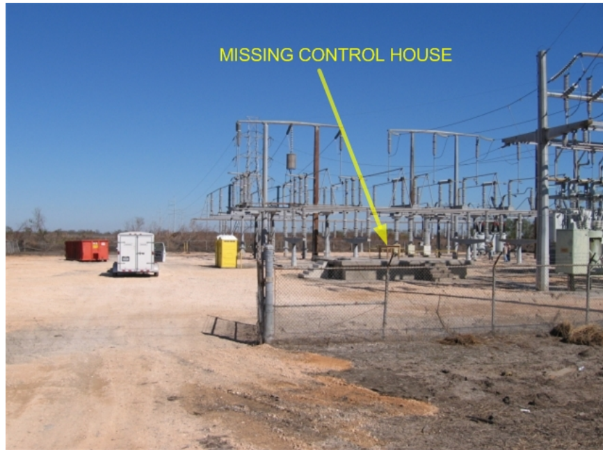
Fig. 8.4. Entergy 66MVA Substation near Belair, LA
