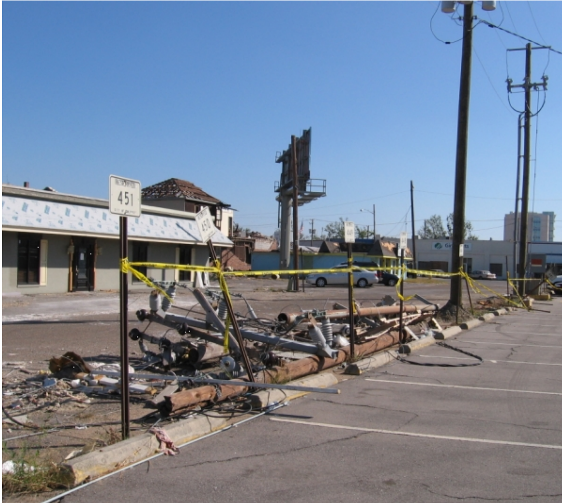
Fig. 3.20. Broken electrical pole in Biloxi, MS
