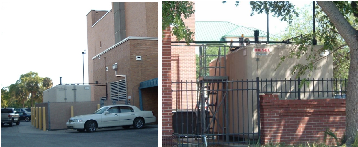
Fig. 5.76. Verizon CO fuel tanks on the Gulf Coast, Left: Sarasota, Florida, Right: 8000 gallon tank of Ybor city CO, Tampa, Florida
