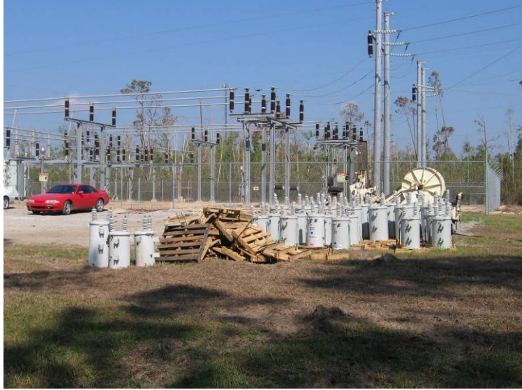
Fig. 8.12. Staged distribution transformers
