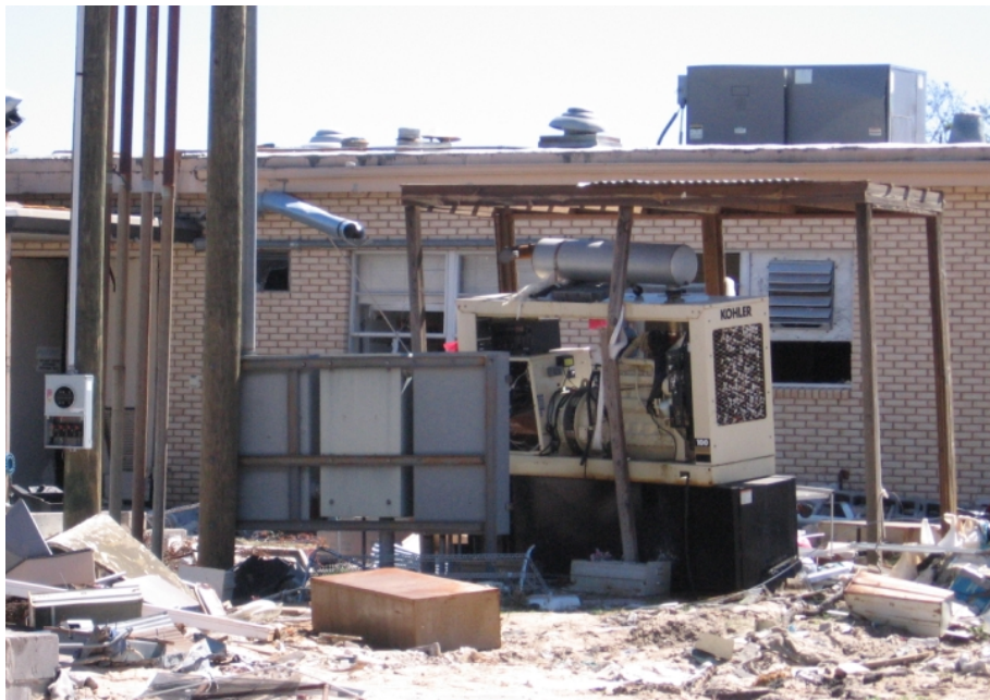
Fig. 9.7. Destroyed genset at nursing home in Pass Christian, MS
