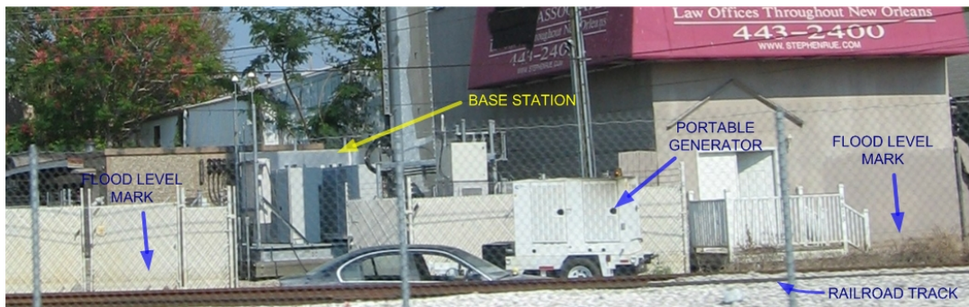
Fig. 6.47. Cell site in New Orleans, northwest of downtown
