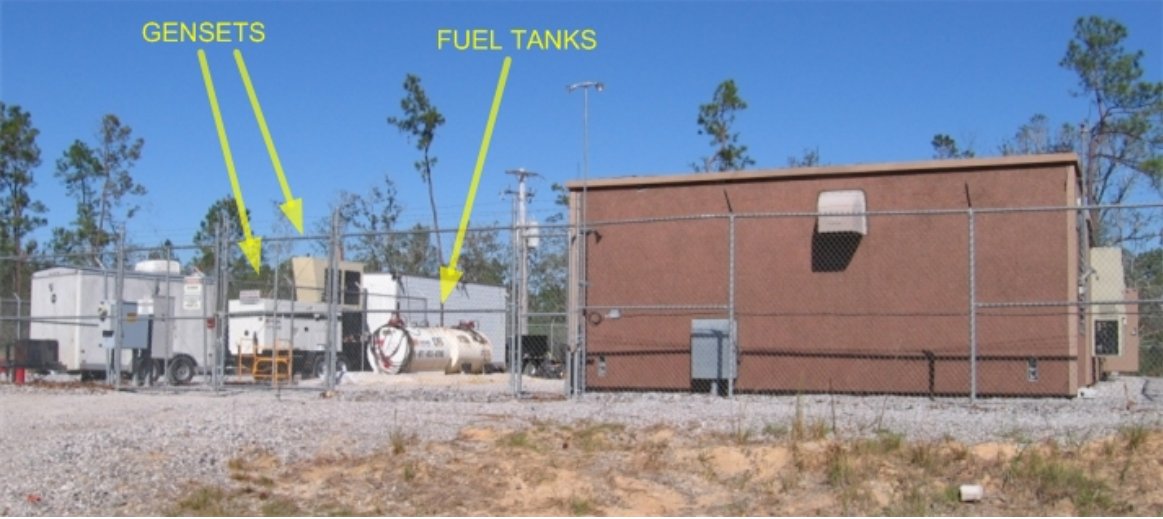
Fig. 5.81. Level3 Communications transmission site south of Pearlinton, Mississippi
