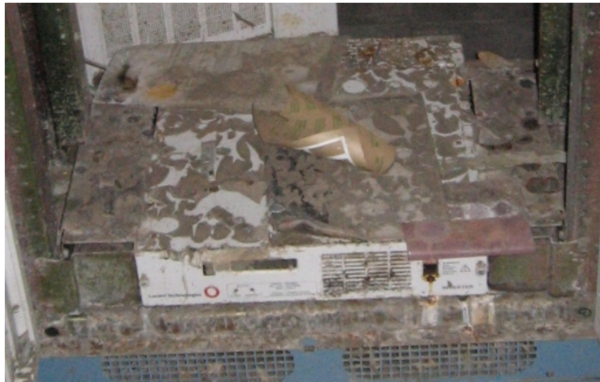
Fig. 4.2. Inverter with mud
