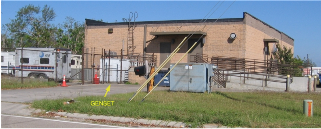
Fig. 5.79. AT&T regeneration site in Gulfport, Mississippi
