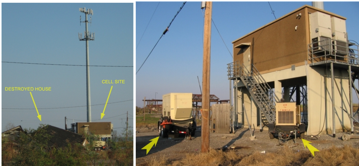
Fig. 6.42. (a) General view of the north cell site in Irish Bayou, (b) Closer view of the same site with two portable generators indicated by yellow arrows
