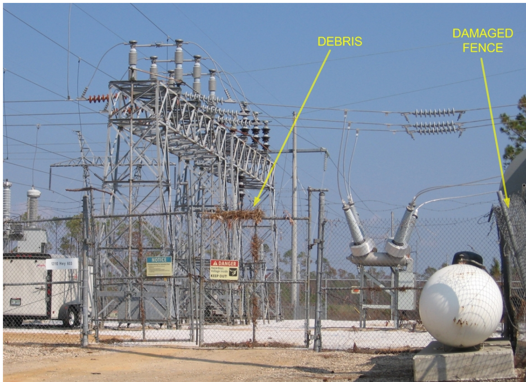
Fig. 8.5. Damaged substation on Route 603, northwest of Waveland, MS
