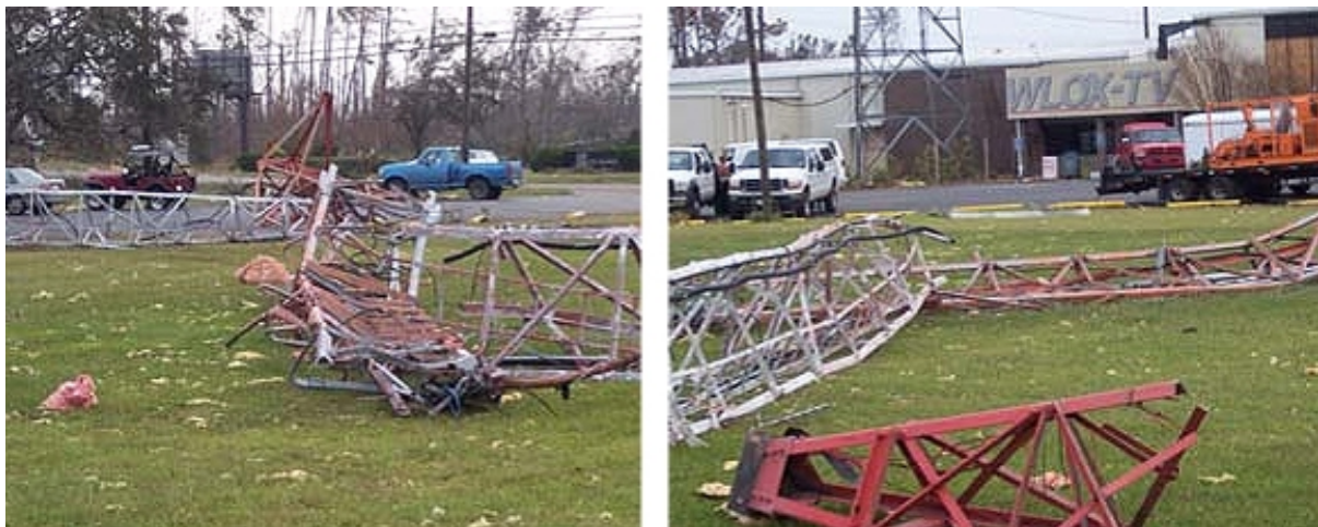
Fig. 7.3. WLOX-TV antenna tower [36]
