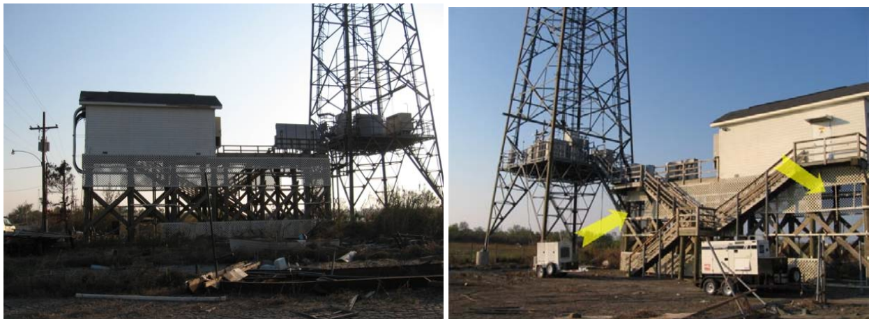
Fig. 6.40. (a) North side of cell site in Irish Bayou, (b) South side of the same site with arrows indicating the maximum height reached by the storm surge
