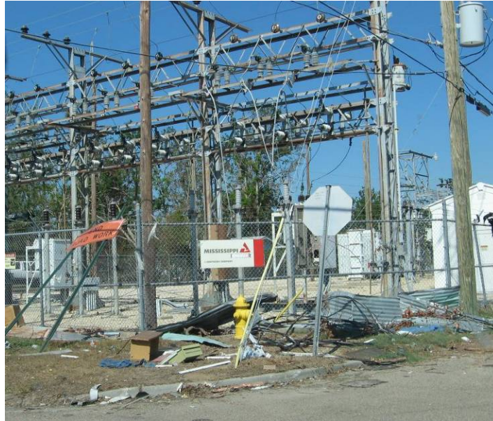
Fig. 8.9. Mississippi Power substation in Biloxi, MS
