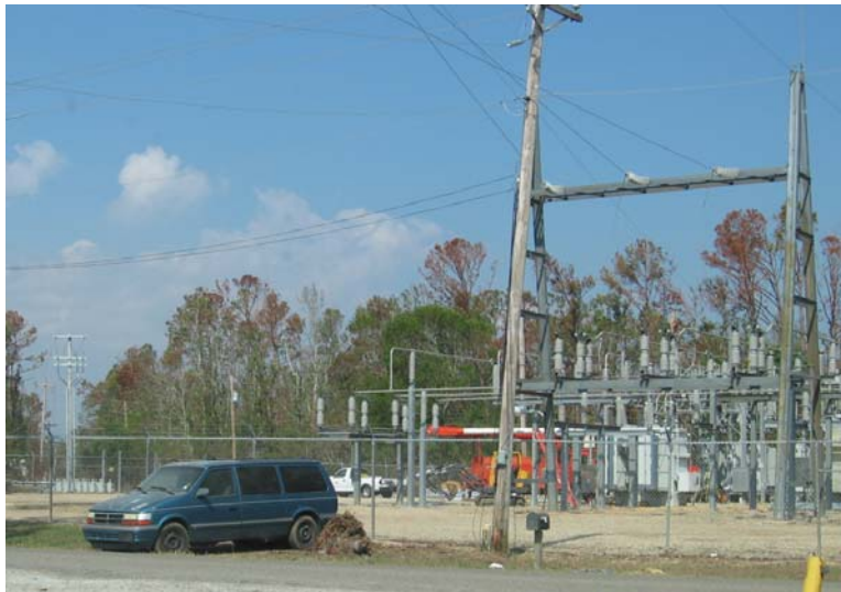
Fig. 8.6. Substation in Waveland, MS
