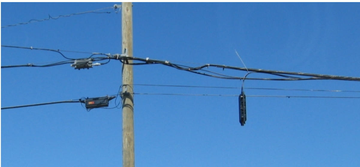
Fig. 3.21. Damaged CATV fiber-optic cable
