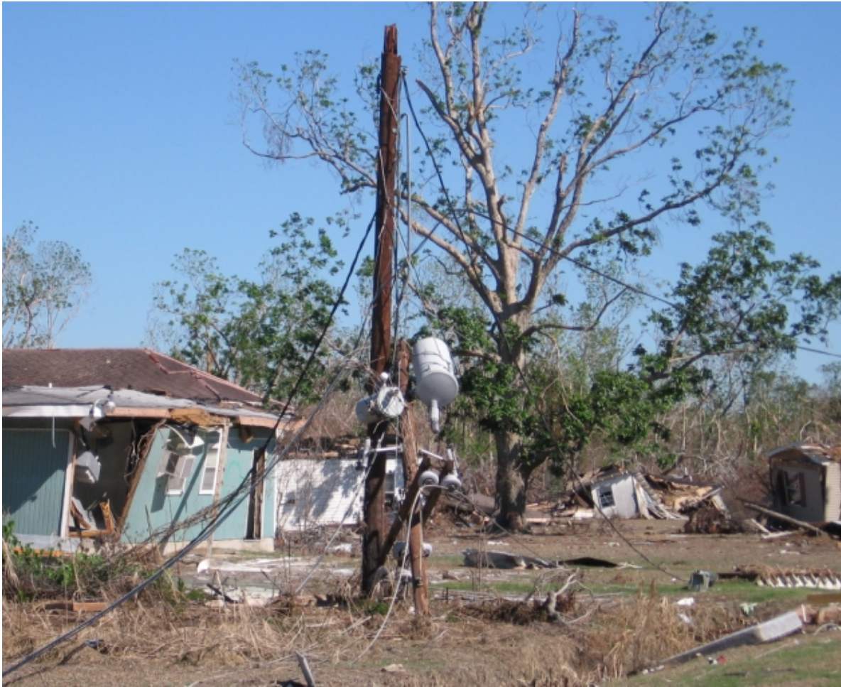
Fig. 3.3. Severe structural damage to houses and a broken pole with distribution transformer and telecom outside plant cables in Point A La Hache, LA
