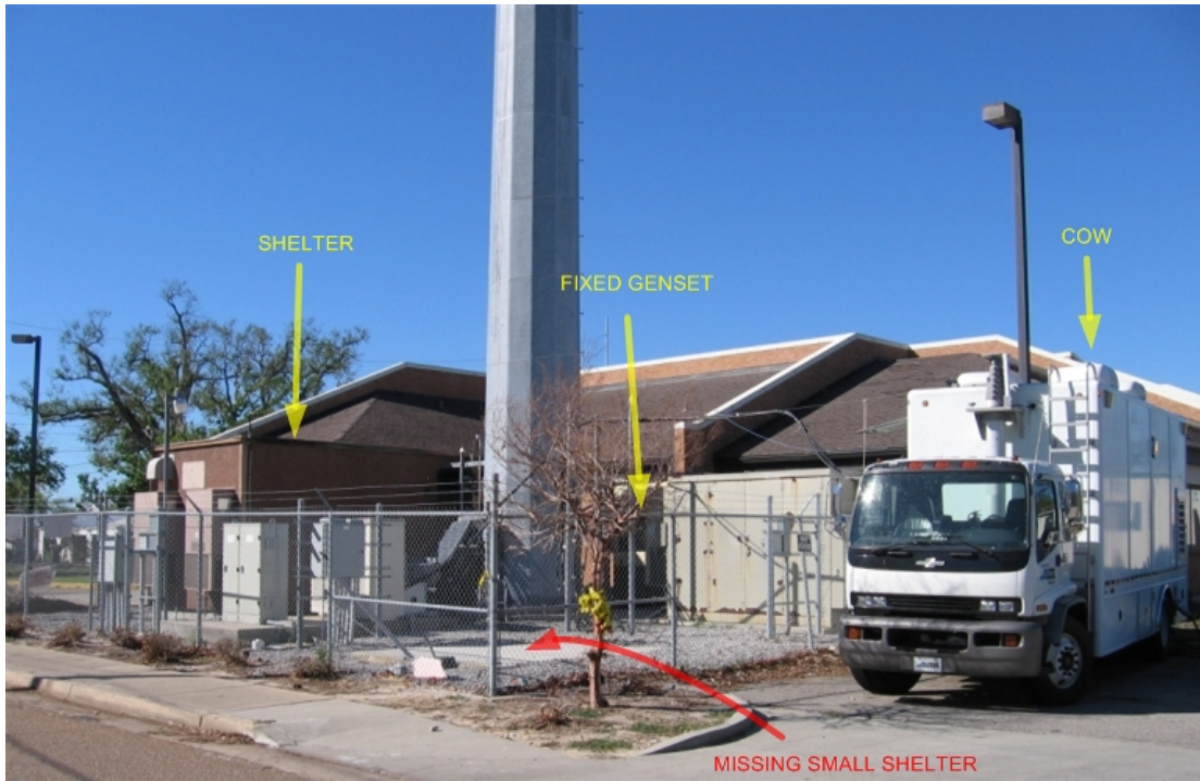
Fig. 6.30. Cell site in Biloxi showing a COW and a missing small shelter
