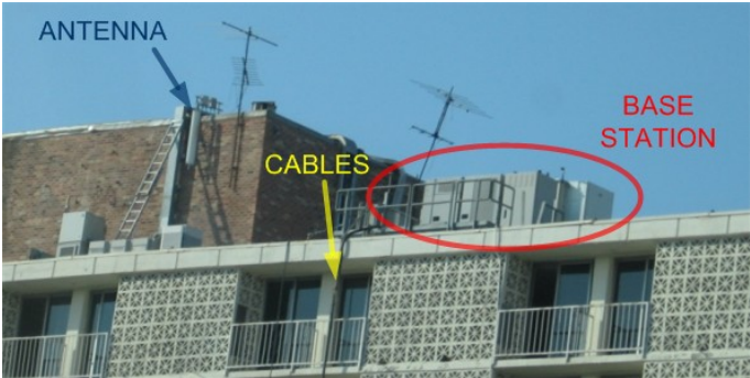
Fig. 6.45. Cell site located on the rooftop in Orleans Parish
