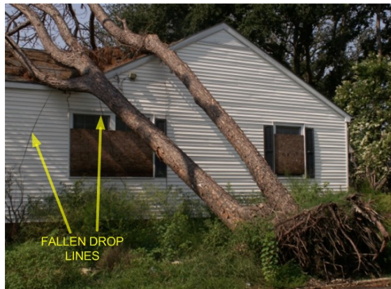
Fig. 10.2 Residence that still shows heavy storm damage from Katrina, July 2006. Photo courtesy of D. Dickey.
