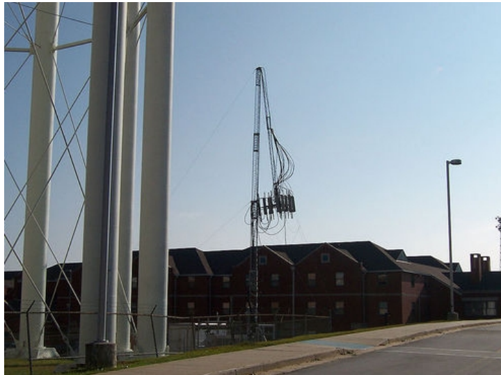
Fig. 6.67. Broken cell-site tower on the Jackson State University campus [38]
