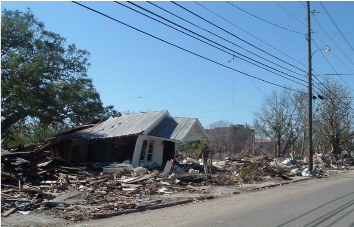
Fig. 3.7. Severe residential damage; none to electrical and PSTN distribution cables in Biloxi, MS
