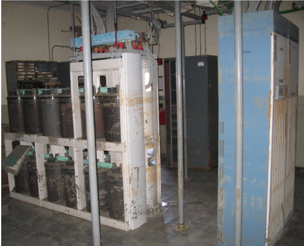
Fig. 4.6. Batteries on the left and rectifier bays on the right, both covered with mud
