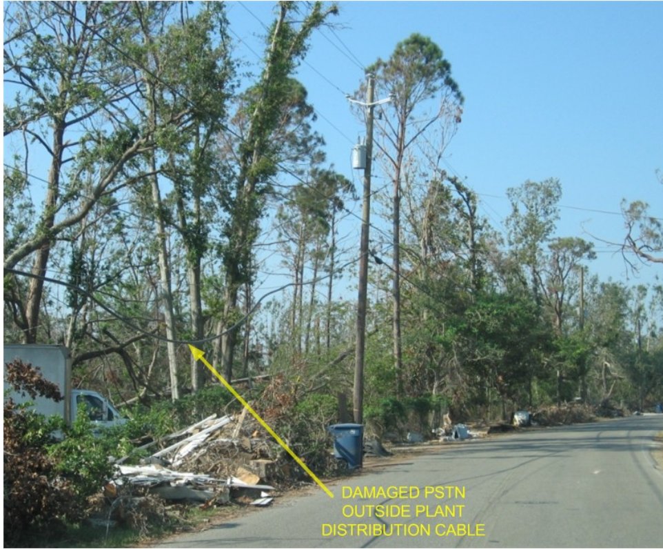
Fig. 3.22. Hanging damaged PSTN outside plant distribution cable
