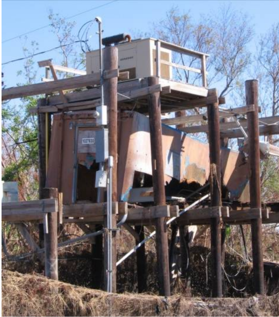
Fig. 7.2. KQLD-FM radio transmitter genset
