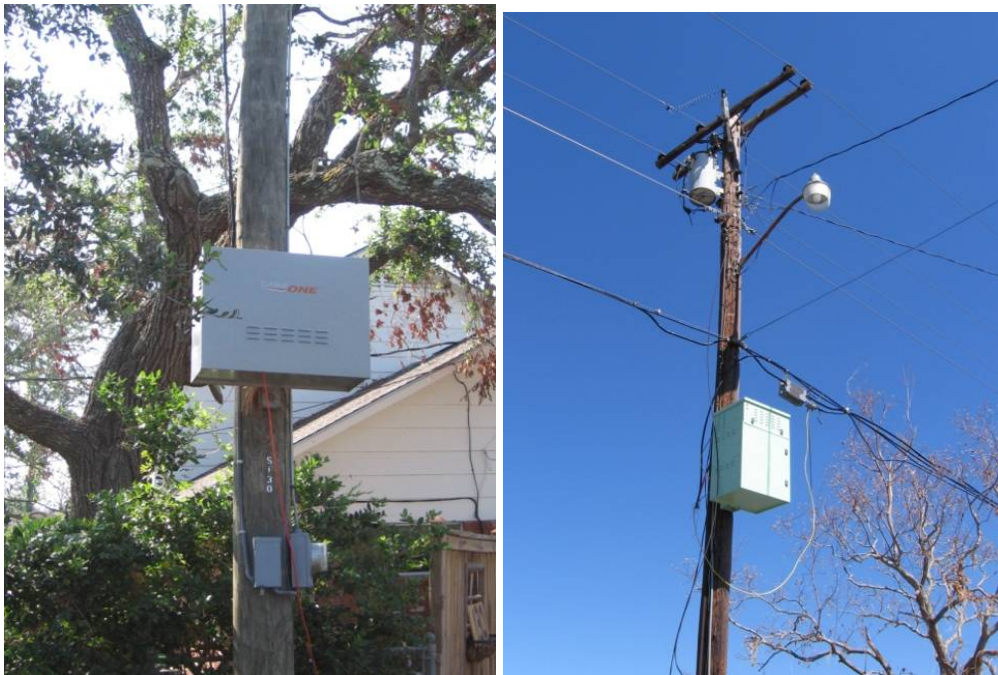
Fig. 7.10. Pole-mounted CATV UPS
