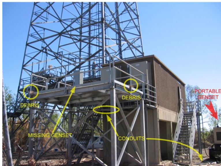
Fig. 6.32. Cell site on highway 46, St. Bernard parish
