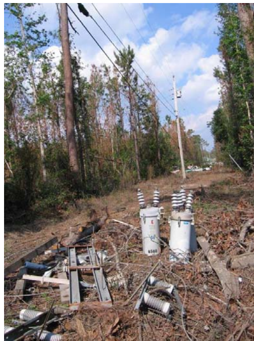
Fig. 8.11. Damaged lines in Pearlington, MS
