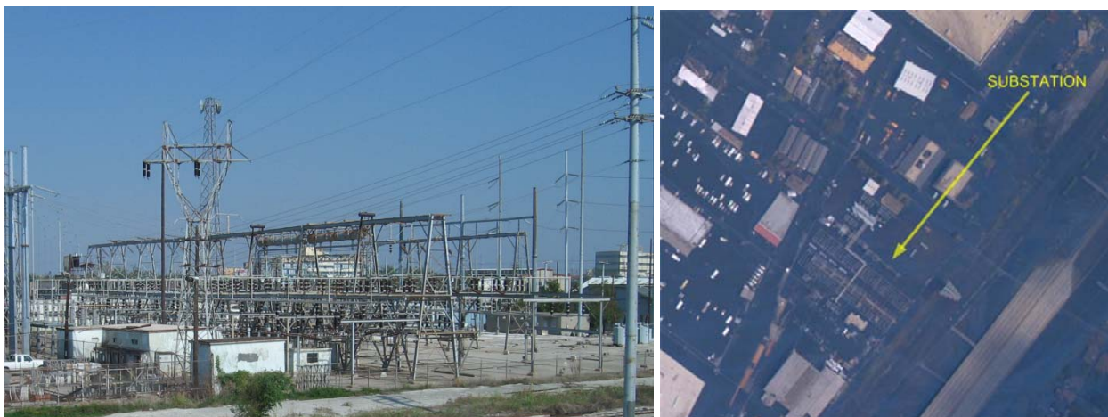
Fig. 8.8. Substation northwest of downtown New Orleans. Aerial view on the right taken on August 31, 2005 [5]
