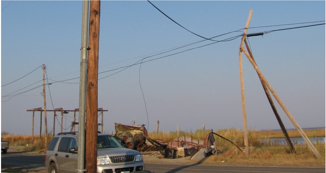
Fig. 3.18. Damaged line on Route 11 south of Lake Pontchartrain, LA
