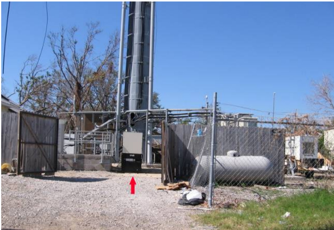
Fig. 6.26. Cell site in Biloxi, MS
