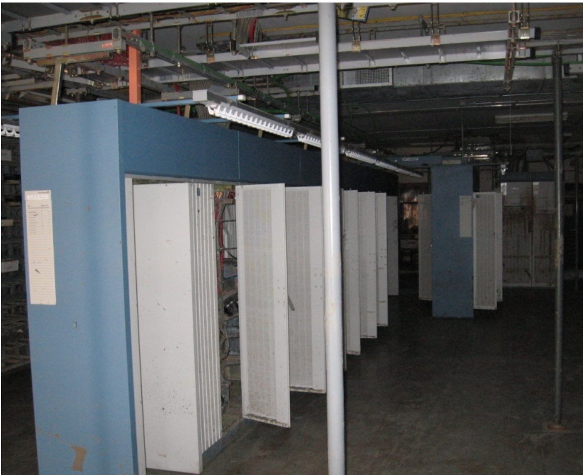
Fig. 4.1. Damaged switch (left). The rectifier bay is in the background, MDF on the left behind the switch. Notice the debris on the cable-racks.
