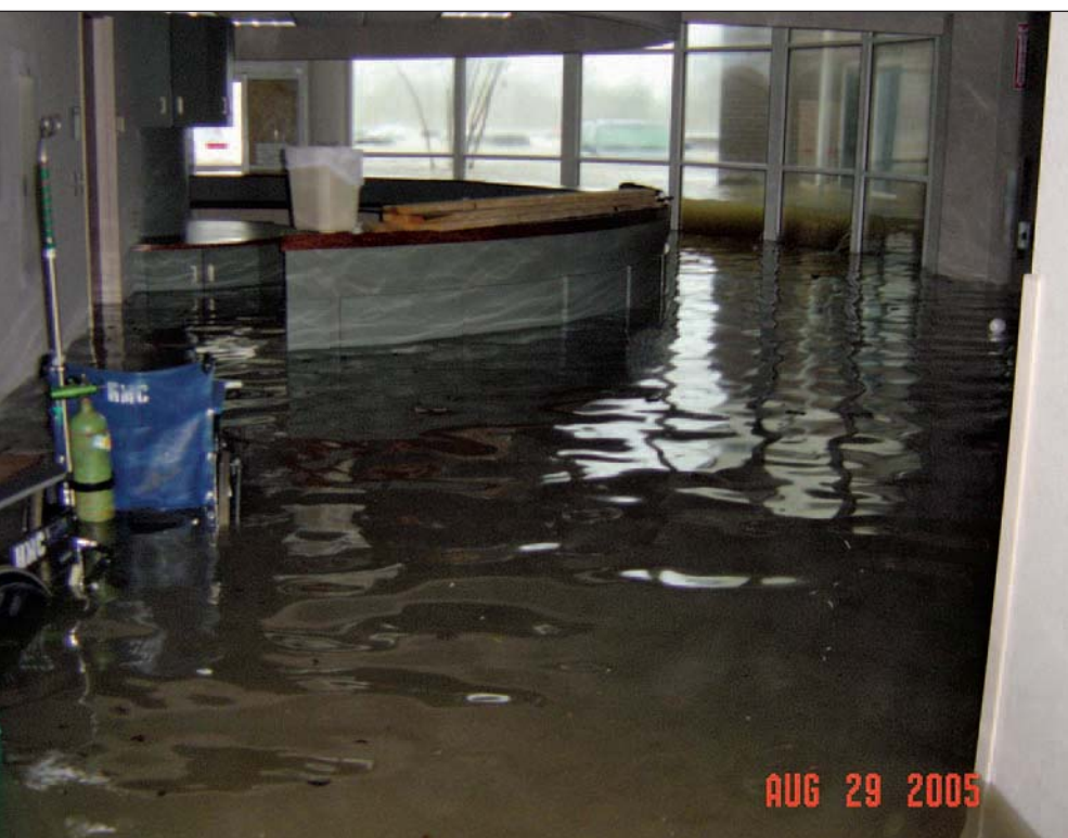
Flooded reception area, Hancock Medical Center, Mississippi Provided to Committee
